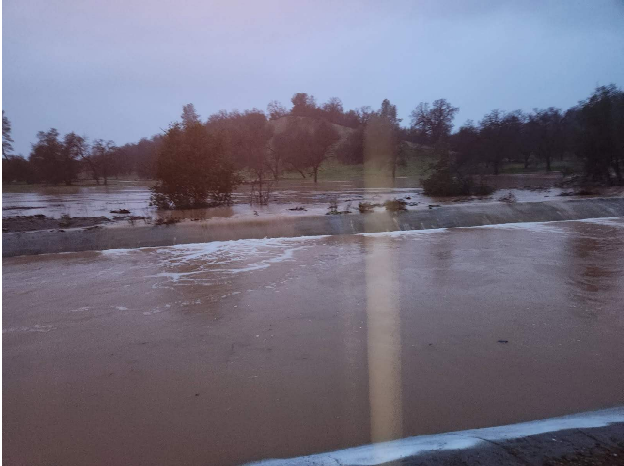
Image 1. Storm Event Breaching Canal Embankment
